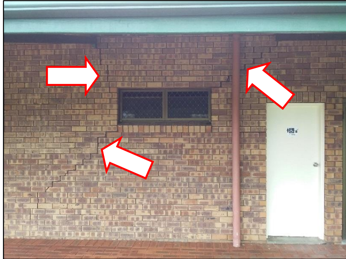
Figure 1 – Cracking to external walls of changeroom, southern side
