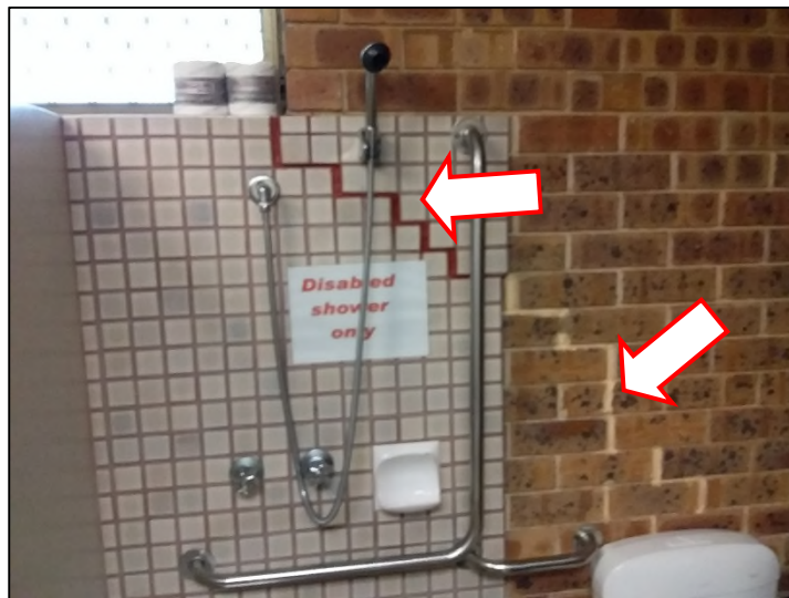
Figure 2 – Cracking to internal leaf of wall shown in figure 1 (Female Changeroom)
