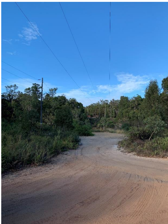
Image 1: Existing Western Power Aerial Cabling
