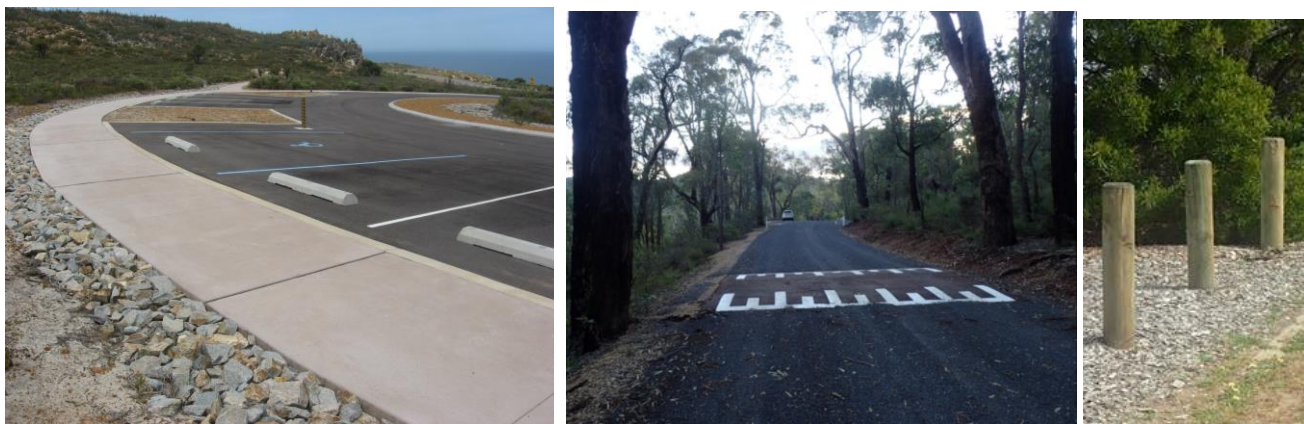
Figure 28: L: Typical parking with black asphalt, wheel stops and concrete collector path C: Low key road construction with speed hump R: Pine bollards
