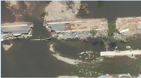
Hillside - Marble Bar Road (severe washout)
